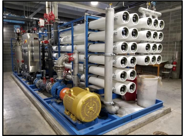
RO Skid in RO Facility
