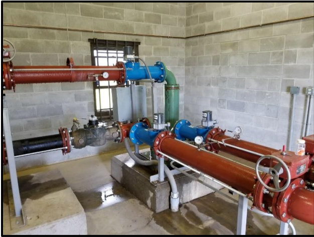
Well 27 Tri-Plex Pump System
