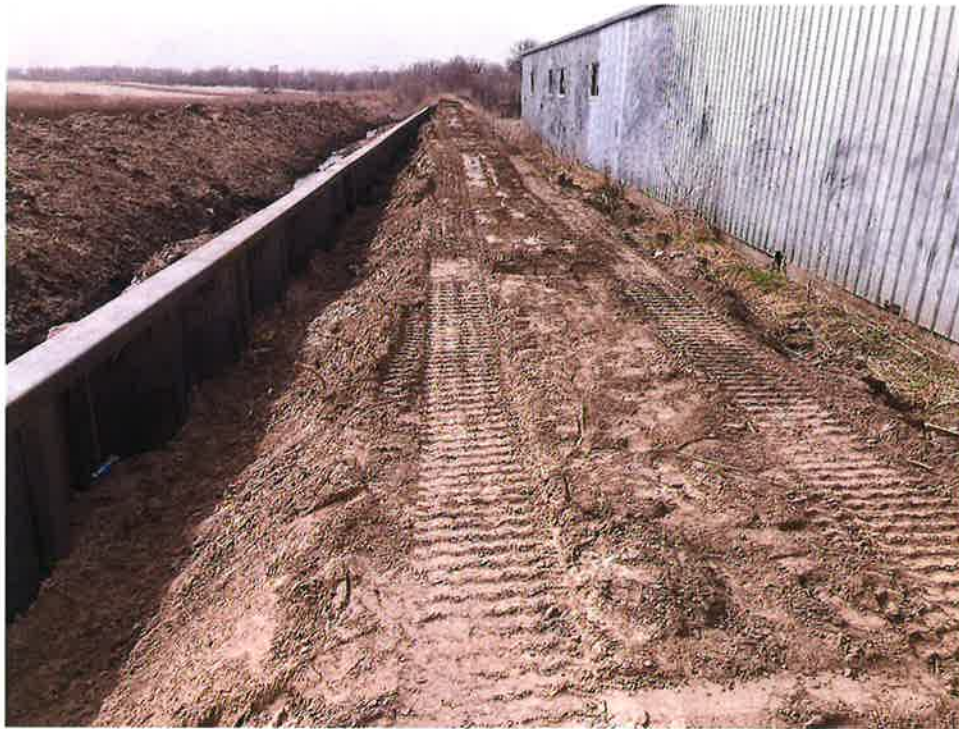
West Point Levee Improvements Construction: Sheet Pile Wall Looking West from Railroad Street
