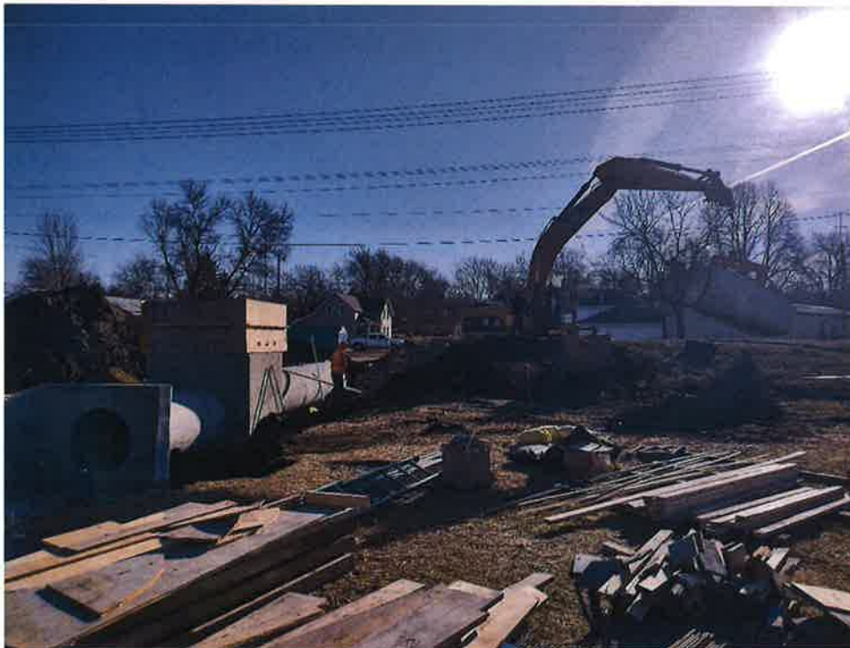
West Point Levee Improvements Construction: New Storm Drainage Outlet Structure at Sta. 19+18
