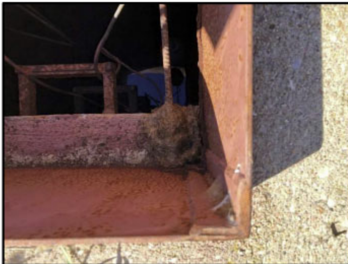
Picture 6: Rust and debris inside the 60,000 gallon tank.
