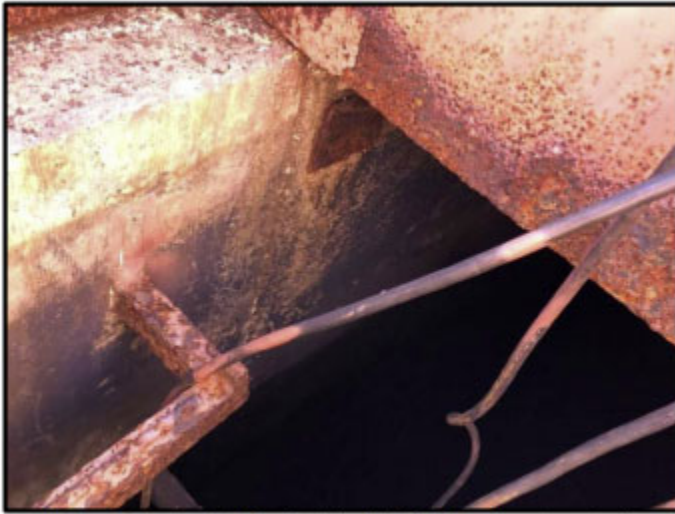
Picture 5: Rust and staining inside of the 60,000 gallon storage tank.
