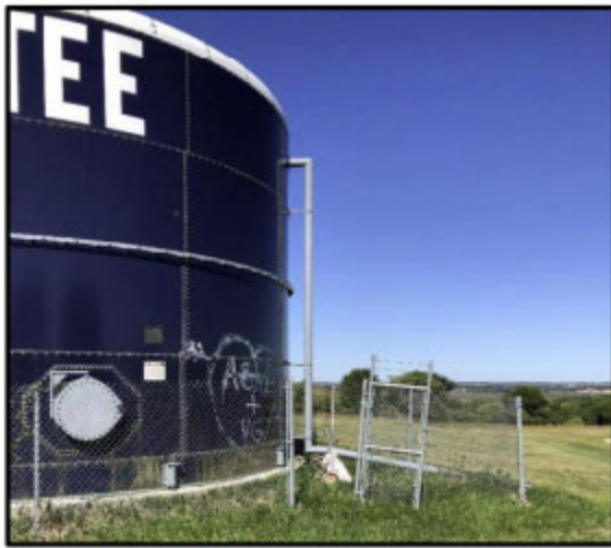
Picture 2: Graffiti on Water Storage Tank.
