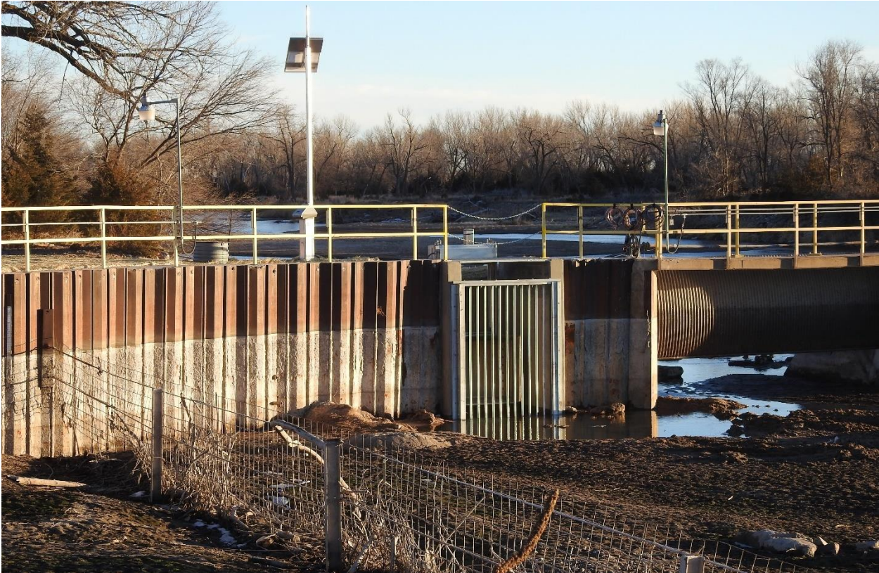
Gothenburg Canal Rubicon gate (upstream view):
