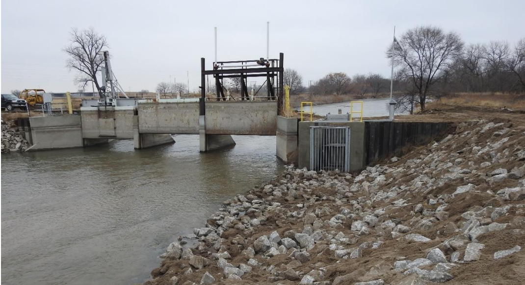
Dawson County Canal Rubicon gate is on the right (upstream view):
