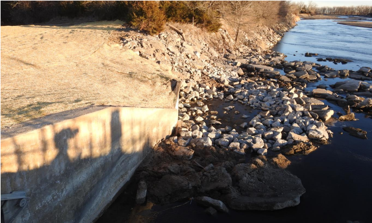
Gothenburg Canal Rubicon gate (downstream view):
