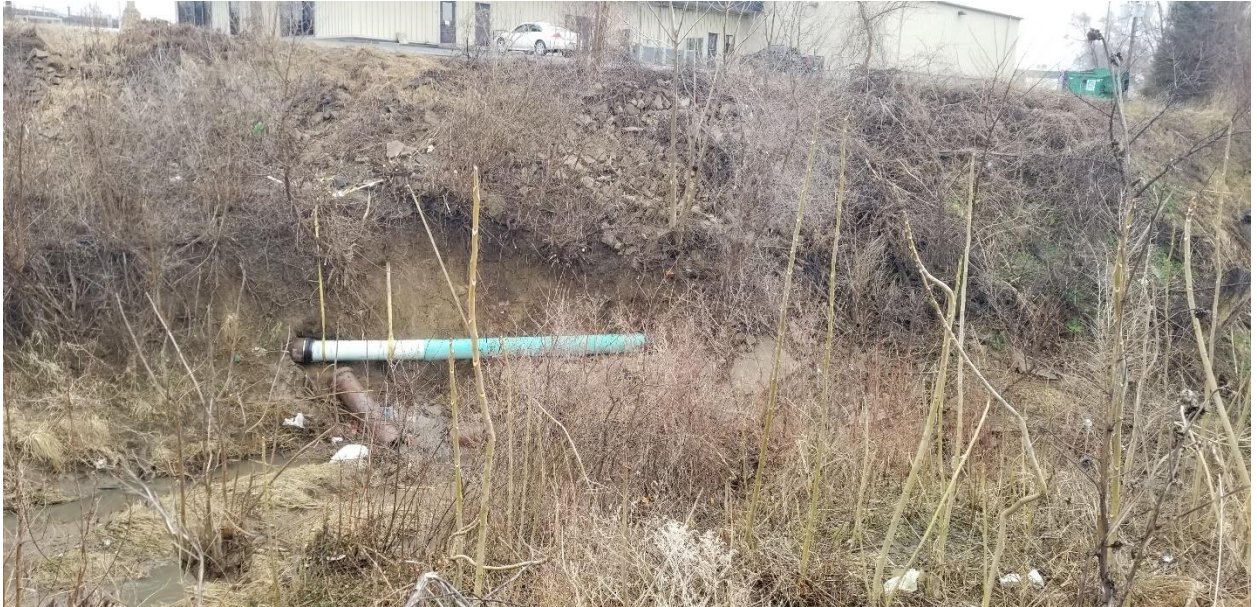
Figure 6: Severe Stream Degradation, Erosion, and a Failed Sanitary Sewer in Omaha
