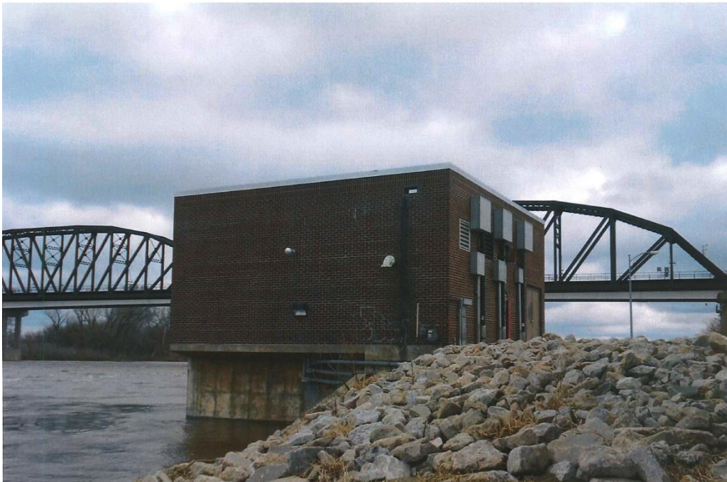
Figure 2 The Blair's water intake pump house on the Missouri River looking downstream toward the Mormon Bridge.
