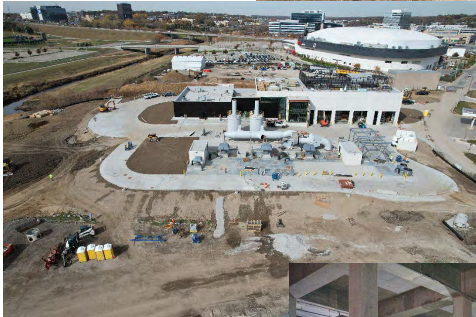
Figure 2 - South Side of the Saddle Creek RTB Facility looking to the North on October 26, 2022 (Courtesy of Multivista)
