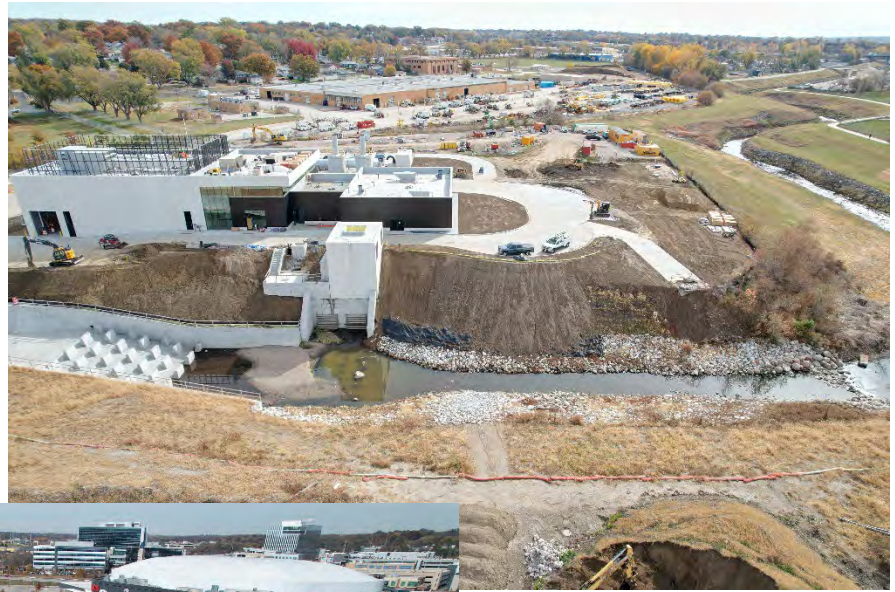
Figure 1 - North Side of the Saddle Creek RTB Facility Looking to the South on October 26, 2022 (Courtesy of Multivista)
