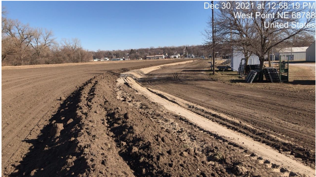
West Point Levee Seepage Berm Construction: Sand Seepage Berm Placed and Top Soiling
