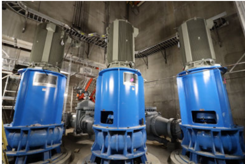
Figure 3-12. Burt Iazard Lift Station New Pumps, Valves, Discharge Piping and Lighting – April 1, 2021
