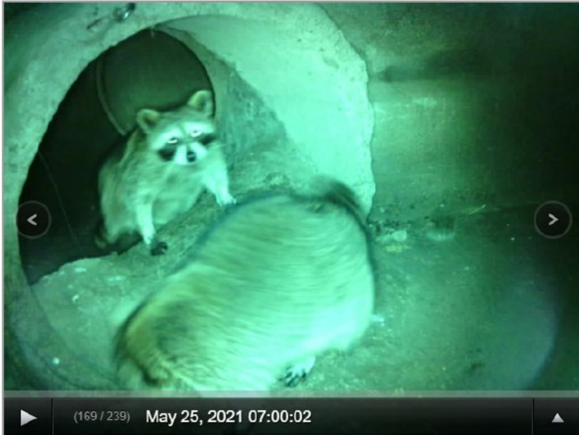
Figure 7-2. Animal Activity on the Weir at CSO 211 (photo courtesy of TREKK Design Group, LLC)
