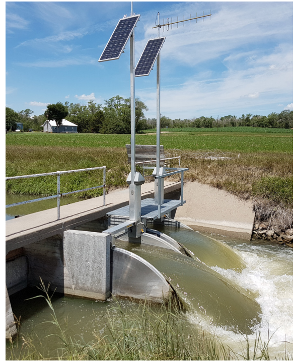
Automated water-tight FlumeGate structure located along the Cambridge Canal.
