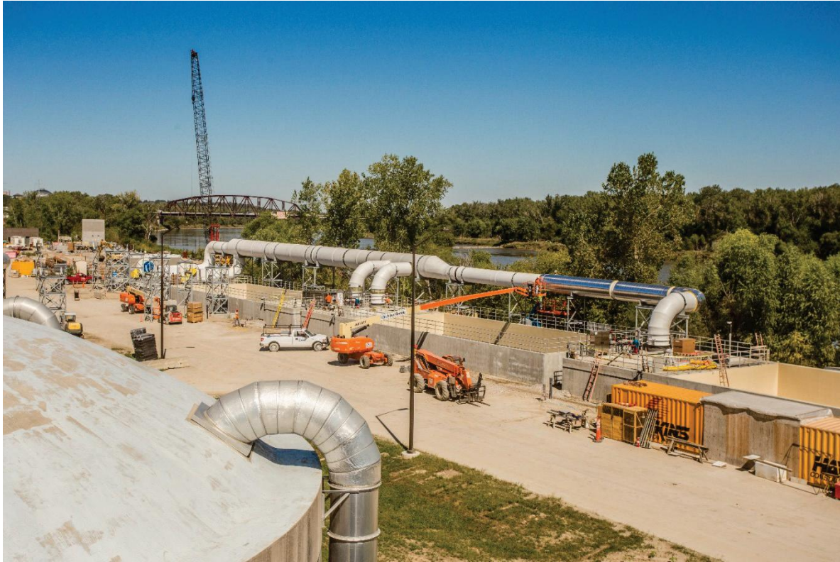
Construction of odor control facilities and ductwork near the south end of the MRWRRF site, looking northeast.
