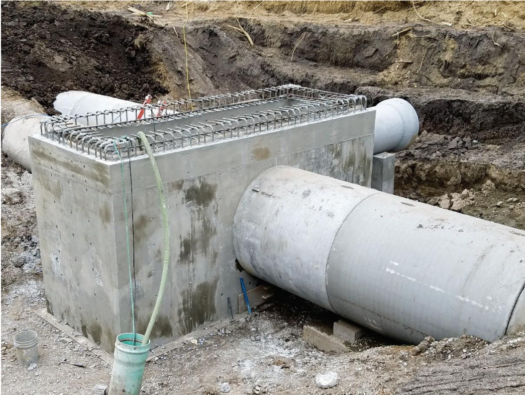
Storm Sewer Junction Structure in Fontenelle Park
