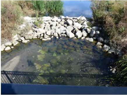
Energy Dissipation Bay
