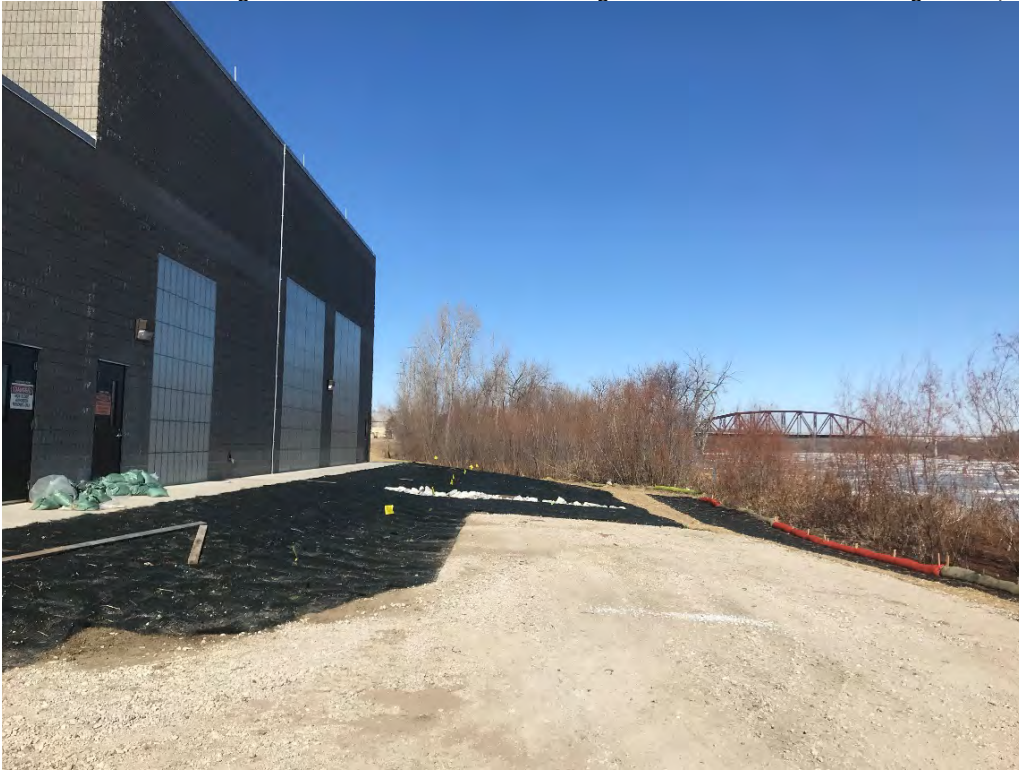
Site Restoration in Progress East of the Chemical Building at the MRWRRF Site, Looking North (Feb. 2020)
