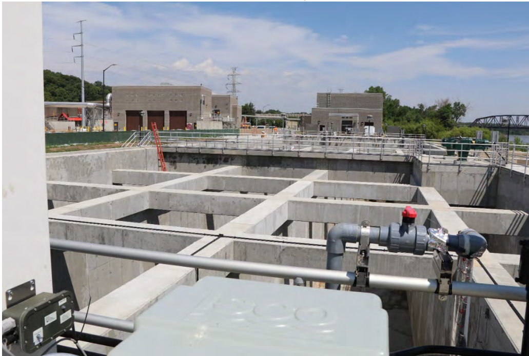
Chlorine Contact Basin at the MRWRRF Site, Looking North (Feb. 2020)
