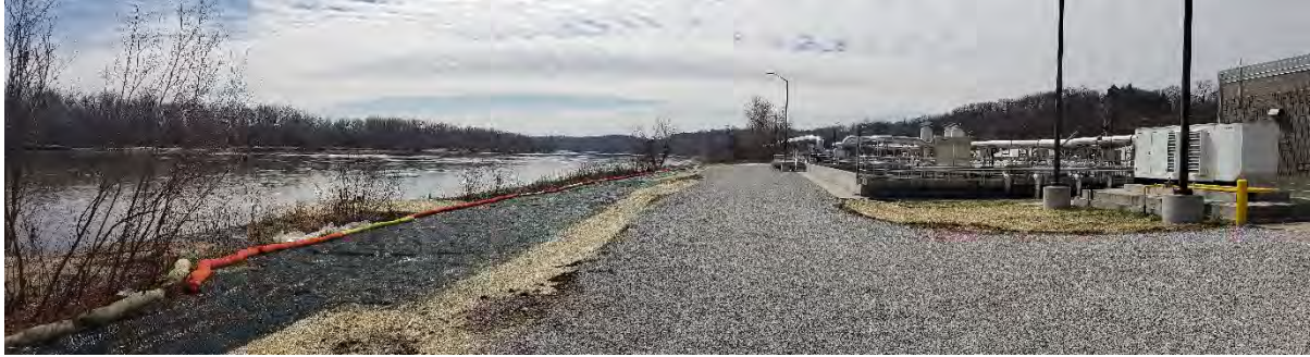
Site restoration in Progress and new access road east of the Chlorine Contact Basin, Looking South (April. 2020)
