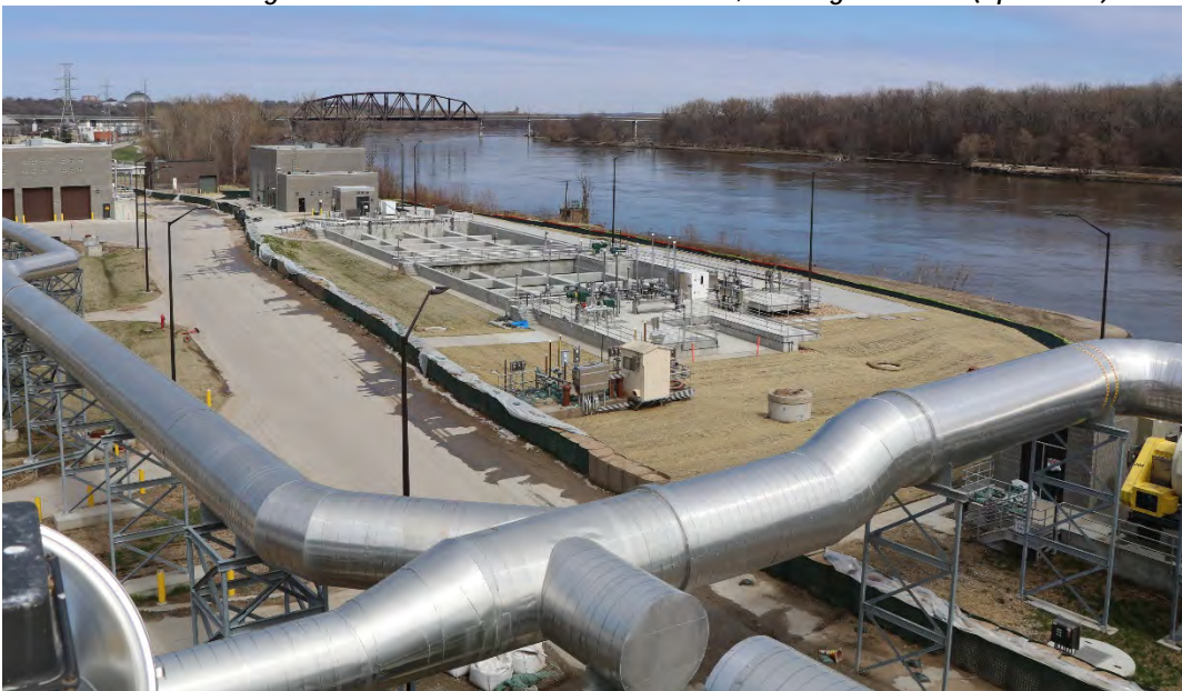
Site Restoration in Progress around the Chlorine Contact Basin, Looking Northeast (April. 2020)
