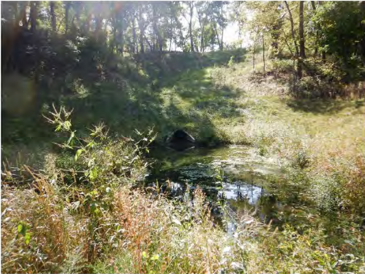
Storm Sewer Outfall into Constructed Wetland in Spring Lake Park, looking up toward 18th and G Streets October 2020
